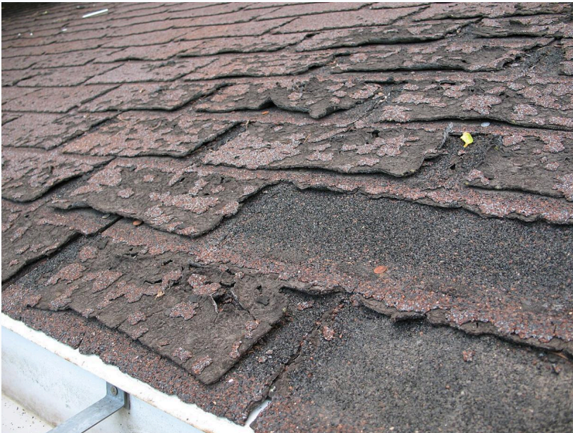
Photo 1: South slope, near ridge
